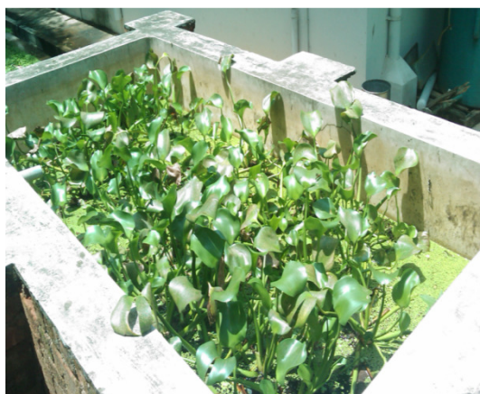
Figure 5.3: Water hyacinth storage tank
