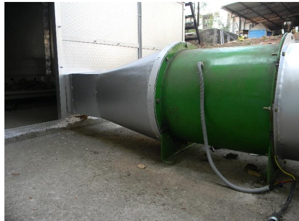
Fig 3.4: Axial blower for combustion air supply.
